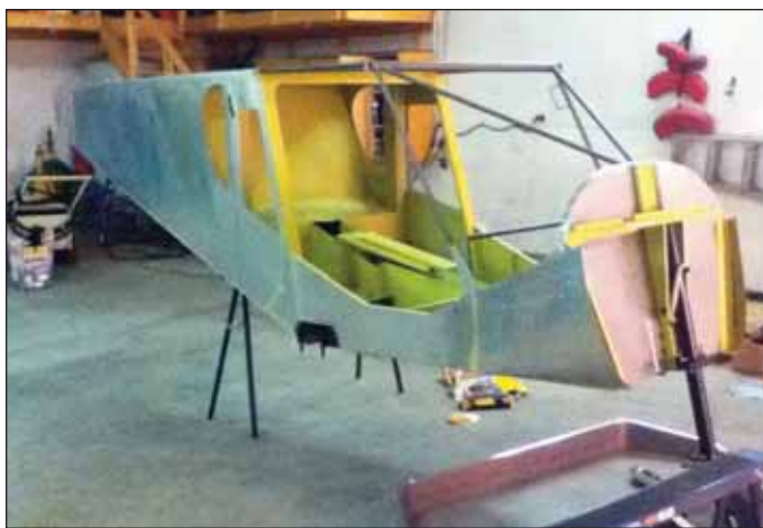
A work in progress – four years to complete from start to finish.
