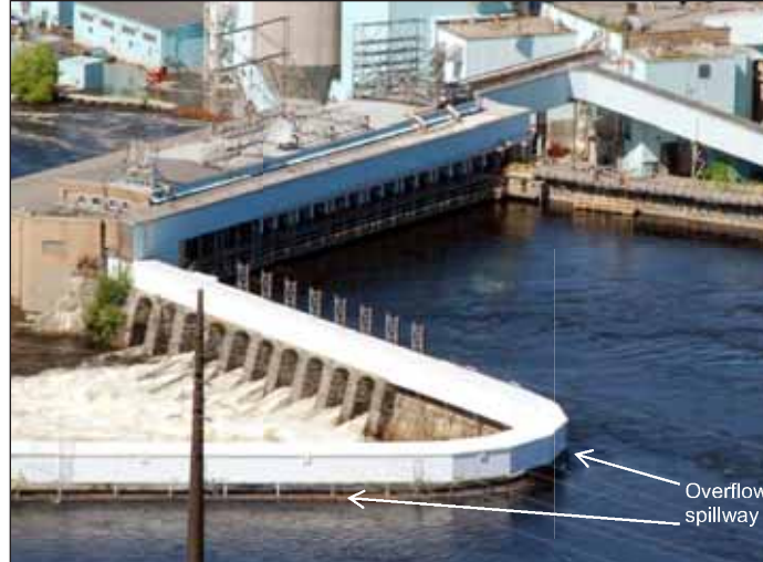
This spillway is designed to safely pass additional flow at high lake levels.
