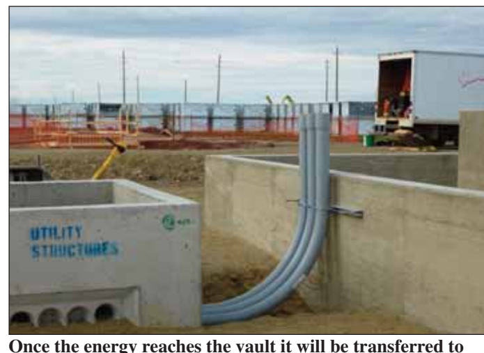
Once the energy reaches the vault it will be transferred to the ON Hydro lines and sent to the distribution centre in Barwick.
