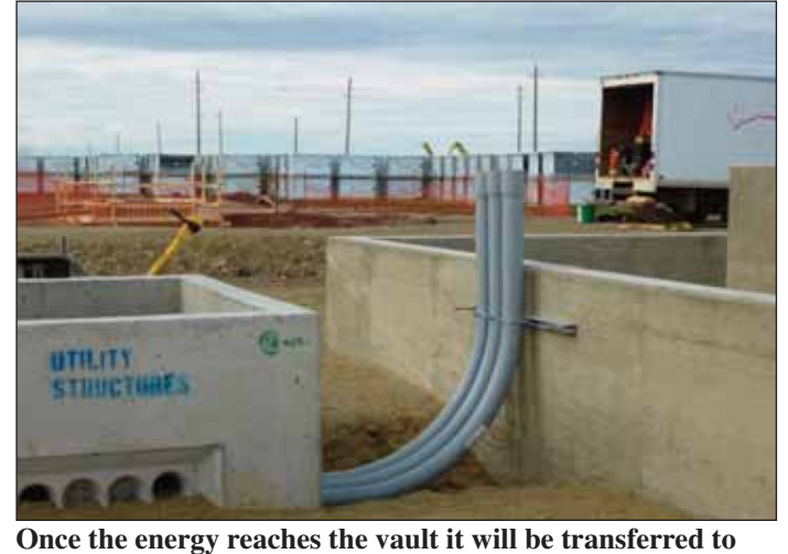
Once the energy reaches the vault it will be transferred to the ON Hydro lines and sent to the distribution centre in Barwick.
